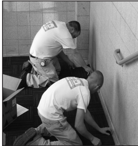
Wilhelm Commercial Builders working on the Druid Hill Y building as a part of the four-month revitalization project.
